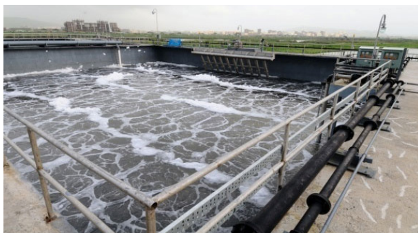
Figure 22.4 A view of sewage treatment plant
